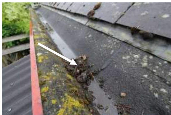
Asbesthoudend mos, in dakgoot
