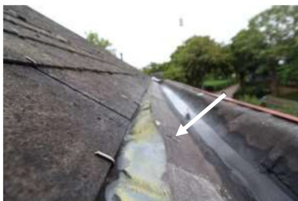
Verontreiniging, hellende daken in dakgoot
