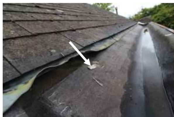
Verontreiniging, hellende daken in dakgoot
